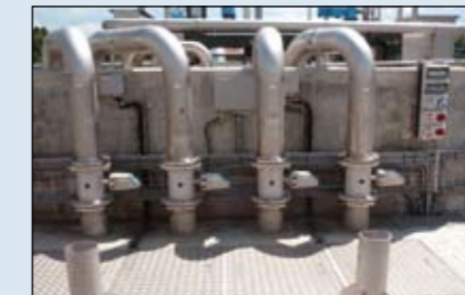
Station de pompage
